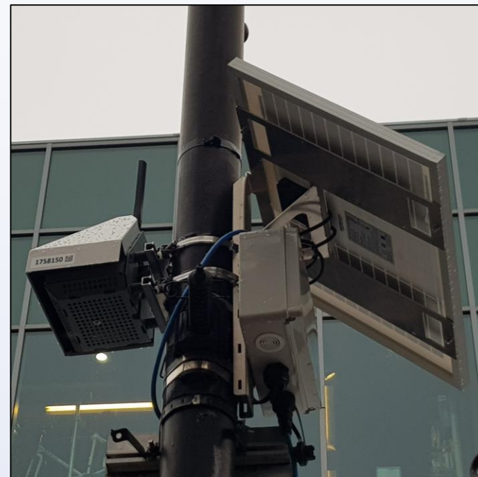
Figure 1: One of the ten air quality sensors located on Northumberland Street.
