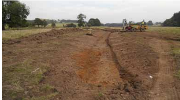
Work underway on the creation of the swale following detailed levels surveys, October 2012.
