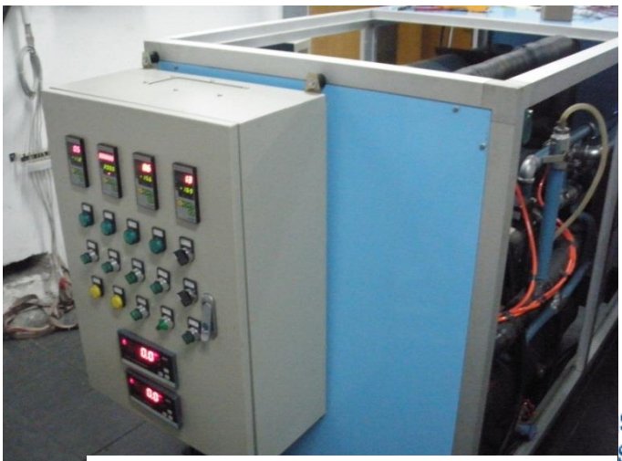
Control panel of chiller
